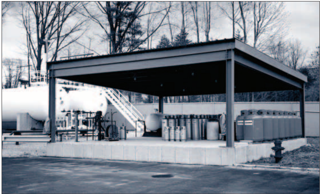
FIGURE 6-12 Cylinder filling station.
