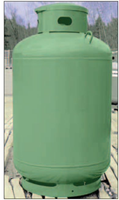
FIGURE 4-10 Stationary cylinder Note: Cylinders are brought to site empty, then filled from a bobtail.
