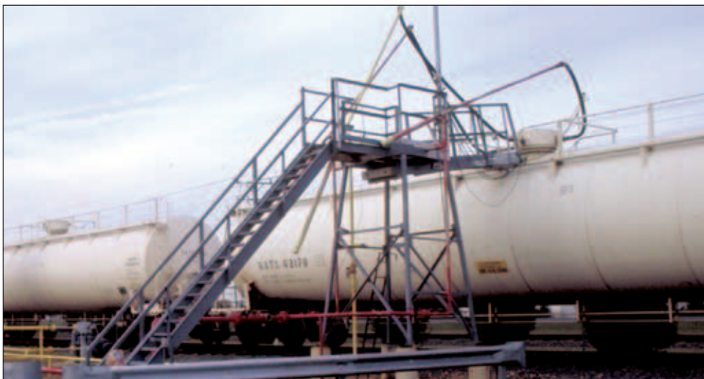
FIGURE 5-19 Propane tank car being off-loaded at a terminal unloading rack.
