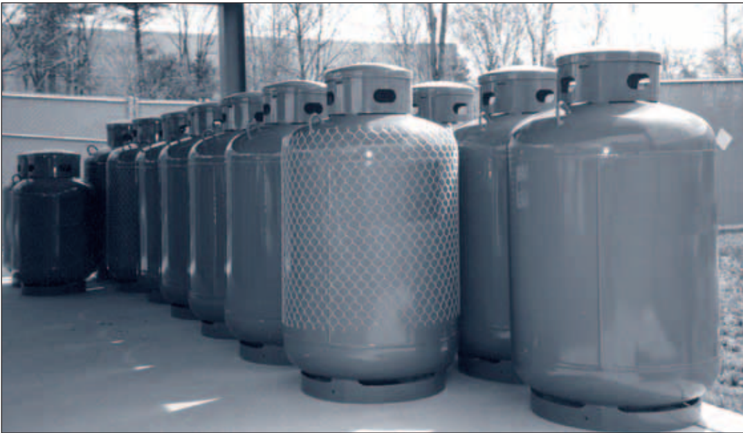
FIGURE 8-13 100 gallon (420 lb.) propane tanks.
