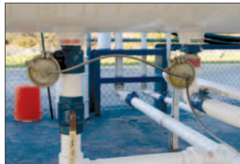
FIGURE 6-4 Internal valve on ASME storage tank.
